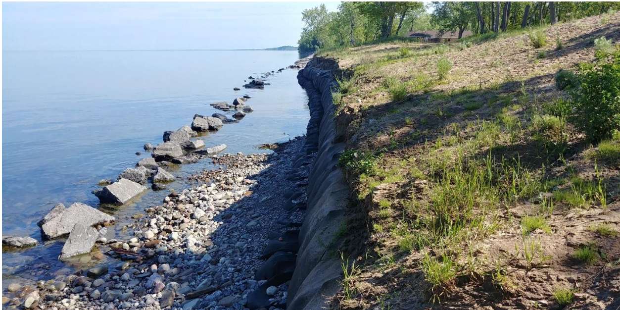
Figure 10. Failed stabilization attempt at Sandy Island Beach, 2019. Here, large, coarse rip-rap was introduced to reduce erosion of an eroding dune face, but deflected and intensified erosion-causing waves into the inadequate upland sediment (not suitable for dune material) resulting in an immediate and excessive loss of shoreline material.
